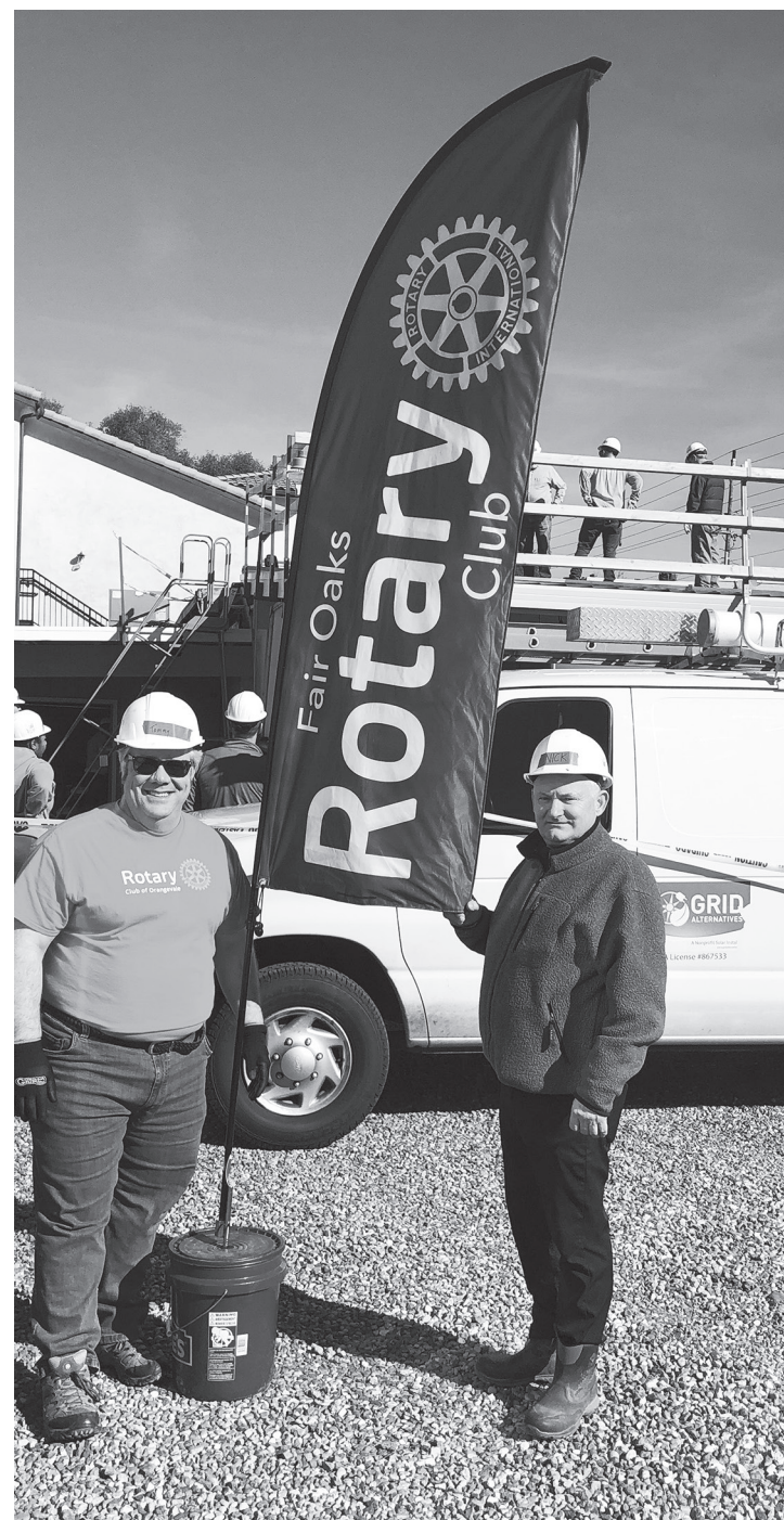
Rotarians Peno and Broad: Orangevale Rotary President Tommy Peno (left) and Fair Oaks Rotarian Nick Broad with Orangevale Food Bank in background and solar crew on roof installing panels.
